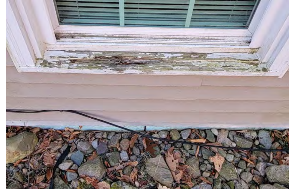
Weathering on Window
